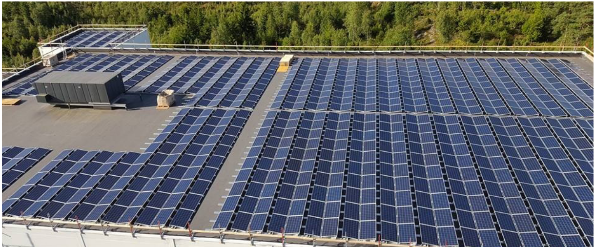
Figure 18 UNILs warehouse at Våler, owned by Norgesgruppen. This system has a rated capacity of approximately 1000kW, similar to the proposed solar energy system for the building at Forus [10].
